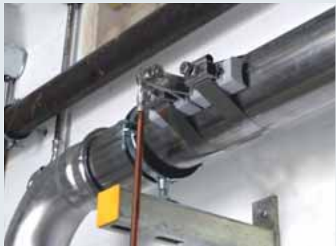
Attached to a StSt pipe
